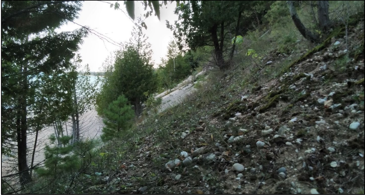
Figure 51. Recent cliff falls can be seen in the steep bluff along the sand and gravel beach (EOID 20444). Photographs taken on September 9, 2022, by Rachel Hackett.
